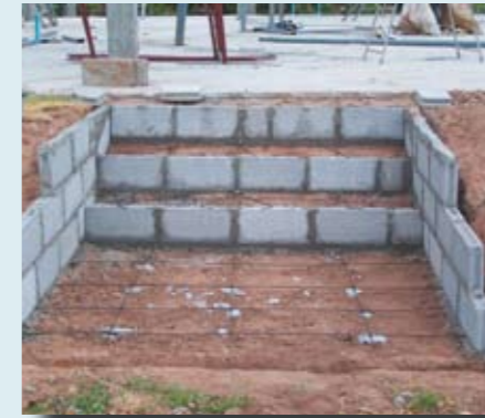
Above: These steps lead up to the kitchen in the new recreation centre.
